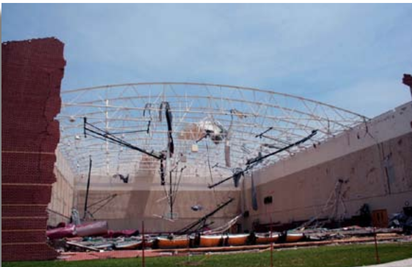
Exterior wall collapsed – no connection at footing
