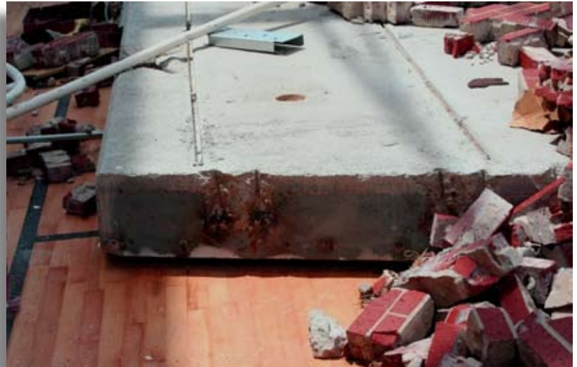
Puddle welded connection on top of wall failed
